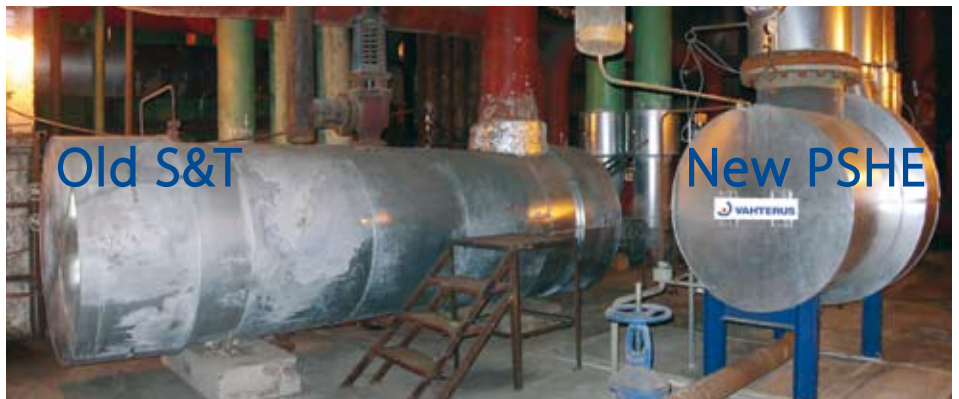
Successful replacement of S&T Heat exchanger in powerplant with significant space saving. 16MW PSHE 9HH-348/1/1 heating district heating water 64°C to 110°C using 0.9bar steam.
