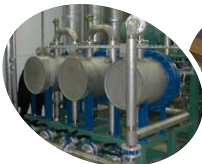
Industrial Heat Pump in Meat Processing Plant
